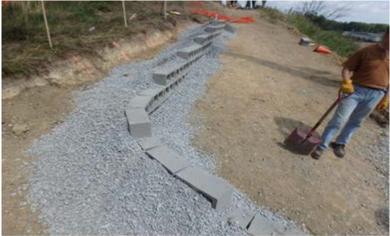
Particular Wall™ made of Concrete Block (Trail Retaining Wall Application -- Northland Library McCandless, PA)
